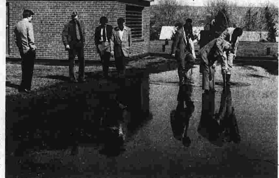
Donald Kuehl, (bending over in the water) measures the depth of the "pool" on top of the Manchester High School roof. Wednesday afternoon as school board members Robert Heavides (left of Kuehl) and Peter Crombie test the water in their rubber boots. Other school officials who were part of group
